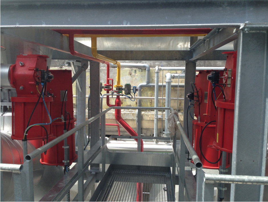
Double Acting Pneumatic Actuators in a solvent recovery plant
